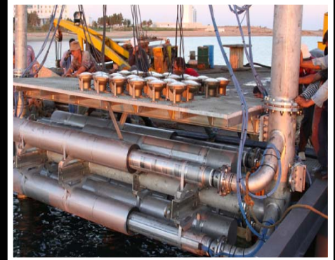
Submersible Pumps with Lights
